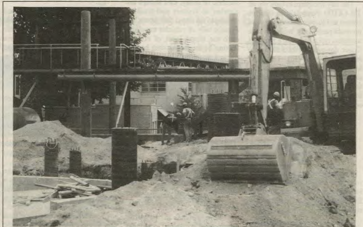
Two weeks ago it looked as though Granville Island's new Waterpark couldn't possibly be completed for its official opening on July 1st, but by now the instant grass is growing nicely and the whole area looks more ship shape with each passing day.
