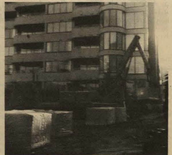
The arm of the pneumatic mobile crane in motion as the operator skilfully unloads the paving blocks.
