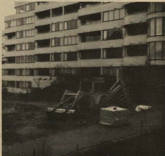
The versatile front and back loader with its grasshopper-like appearance manoeuvres into position to prepare the foundations.
